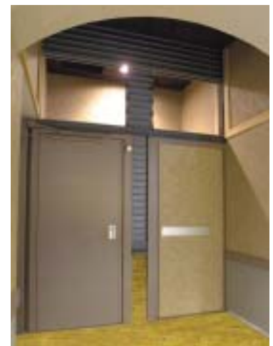
Paradiso Theater's fire door system
