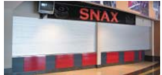
Dillard Door installed Cookson doors in the FedExForum including coiling service doors, counter shutters and security grilles
